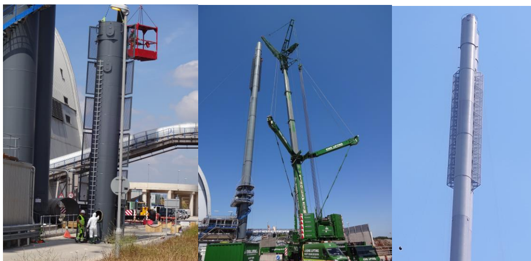
Dampers and side panels at ground level
